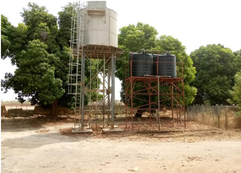
Figure 9: Water tank in Julangel TVET Center
