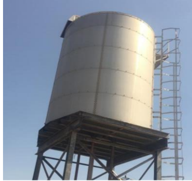
Figure 5.10: Water tank in Kuntaur Health Facility
