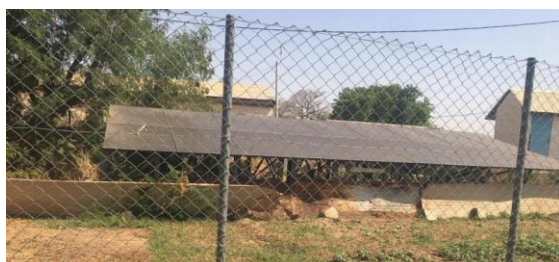
Figure 5.9: Solar PV System in Kuntaur Health Facility
