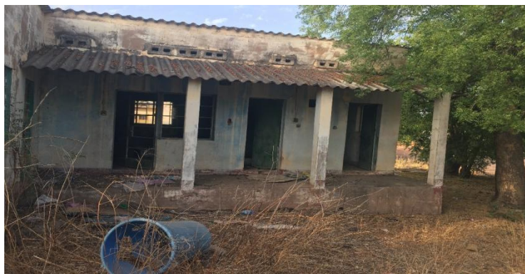
Abandoned staff quarters roofed with asbestos in Fatoto health centre
