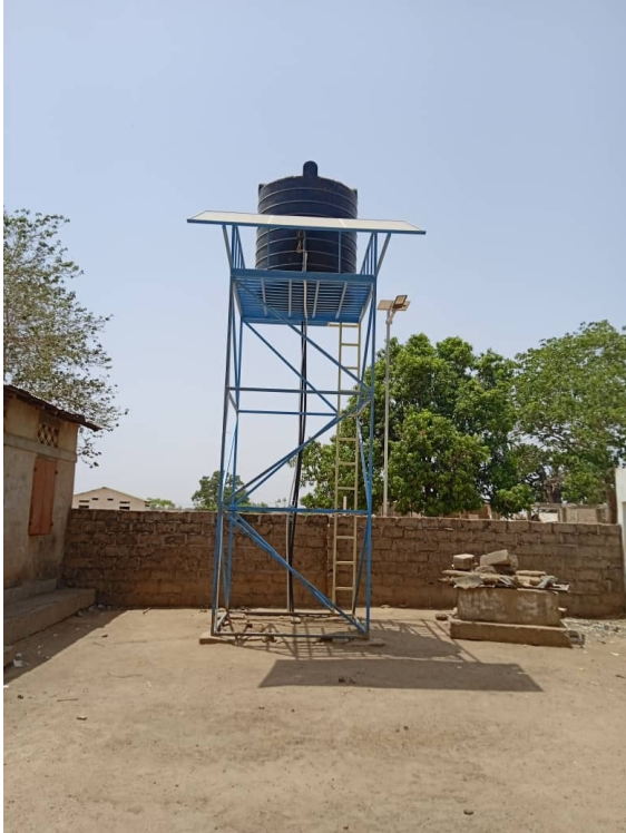
Figure 9: Water tank in Diabugu Batapa ECD Center
