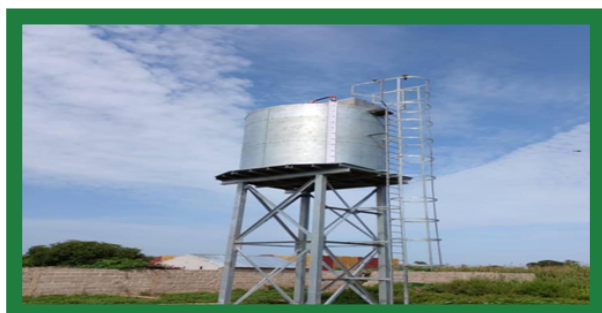
● Overhead tank, Monokoto Keita, Wuli West
